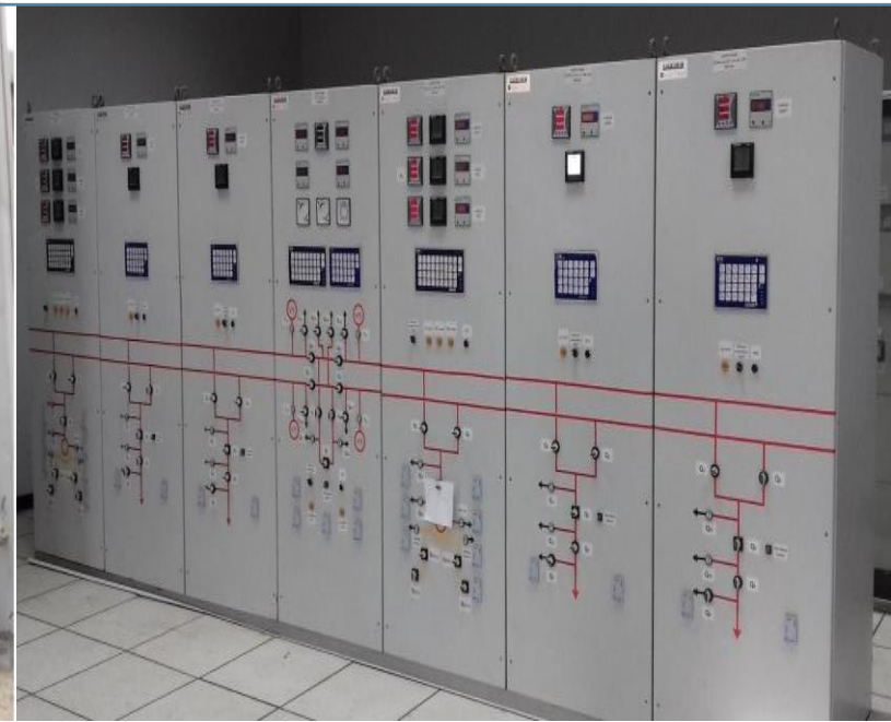
EPS PORT Transformers Substation
